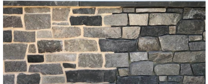
Light vs dark colored mortar joint
